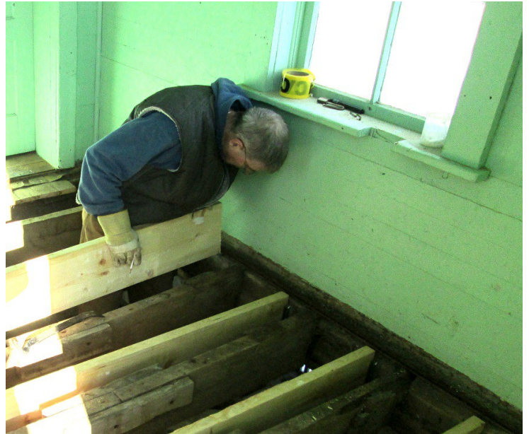
Moore Museum volunteer Dave Beers works to replace floor joists inside the one-room school house.
