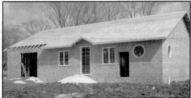
The new Courtright United Church is currently under construction at the corner of Fourth and Main Street.
